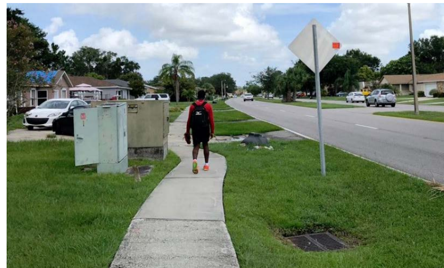
The south side of Buenaventura Boulevard near Royal Palm Drive has an existing 3' to 4' sidewalk.
