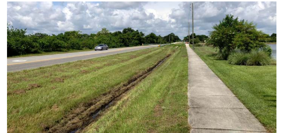
Drainage swale between Partin Settlement Road and the sidewalk, facing west. This condition has been observed scattered along the north side of the roadway for portions of Partin Settlement Road.
