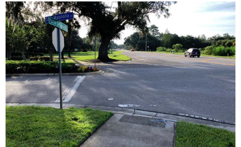
Faded crosswalk markings on the north side of Partin Settlement Road facing east at Star Magnolia Drive. Sidewalk bends around the median island.
