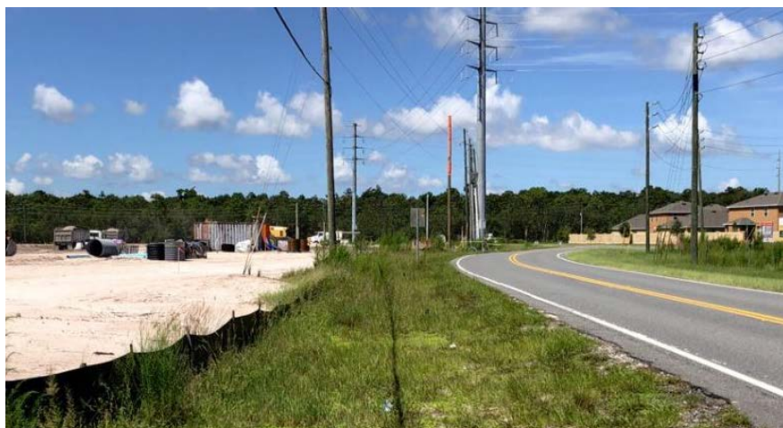
New home construction on south side of Reaves Road at the end of Ham Brown Road, facing west.
