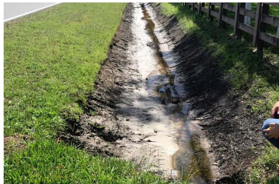
Deep ditch approximately 14-16' on the south side of Reaves Road in front of private property.
