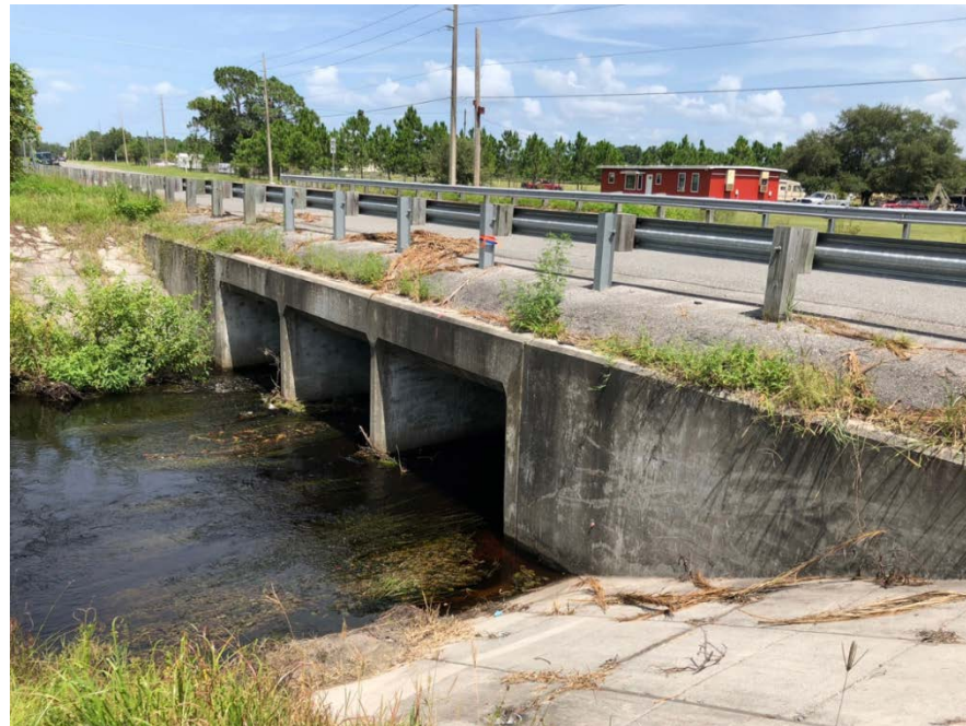
Box culverts under Boggy Creek Road for Jim Branch Creek.
