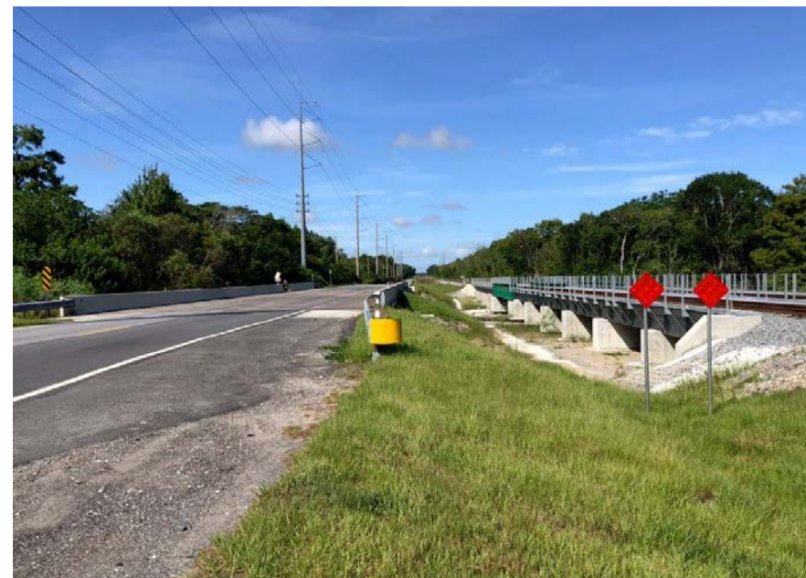
Existing bridge over Shingle Creek. Approximately 40' between bridge walls. Approximately 55' between travel way and Railroad Centerline.
