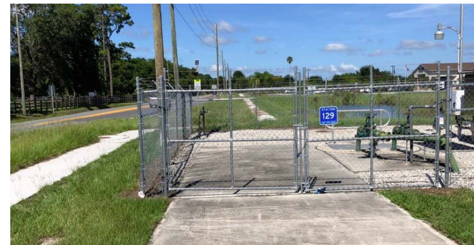
Utility station in apparent right of way path on the north side of Reaves Road.
