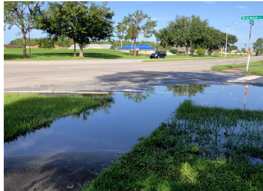
Briarwood Drive drainage issues. At the time of photo there was no recent rain and tadpoles were observed in the water.
