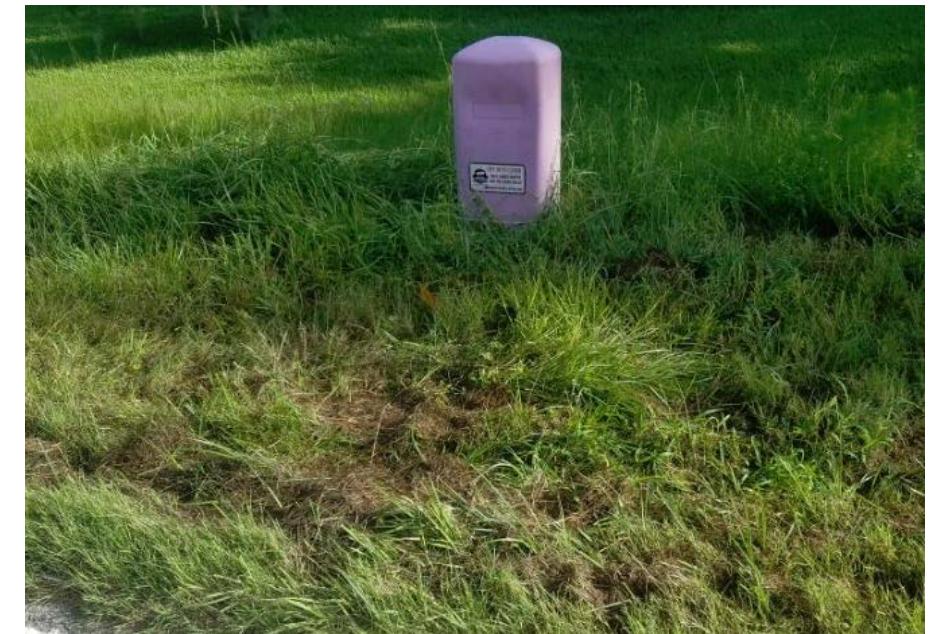
Located on the north side of Partin Settlement Road, 9-foot offset from travel way to reclaimed water valve.
