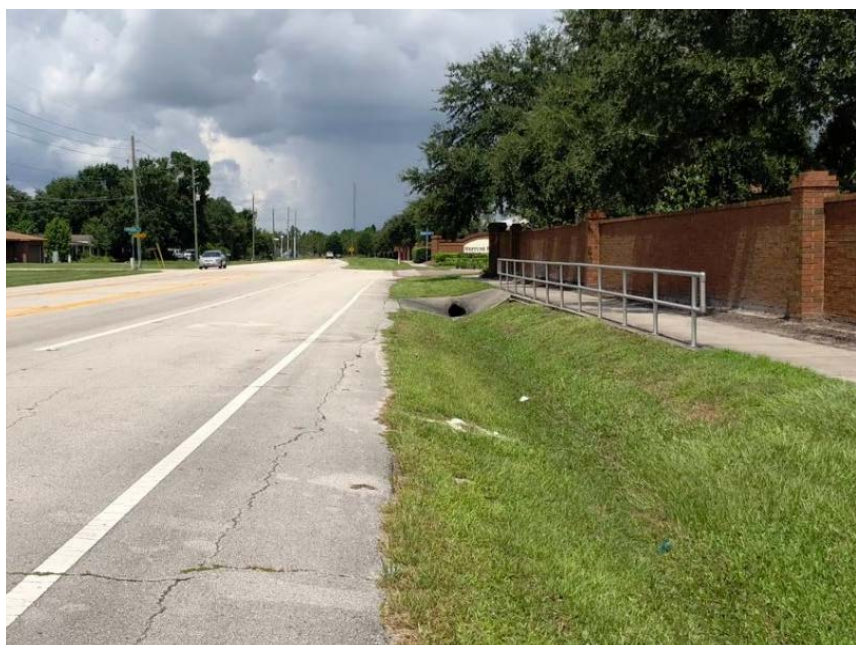
Pedestrian railing between the sidewalk and drainage swale on the north side of Partin Settlement Road. A brick wall for the sub-division is adjacent to the sidewalk minimizing the useable space.
