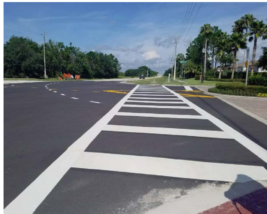
Signalized intersection under construction at Partin Settlement Road and Remington Boulevard, north side of the roadway.
