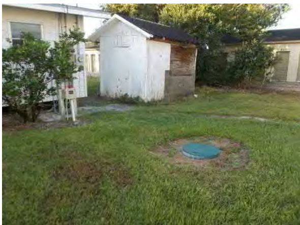
Photo #131 Pond 5(3), Warehouse septic tank.
