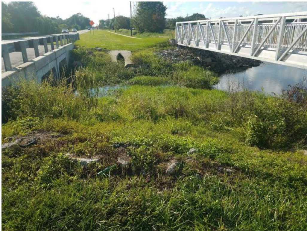
Existing rubble riprap slopes between Partin Settlement Road and Pedestrian bridge. Facing west.
