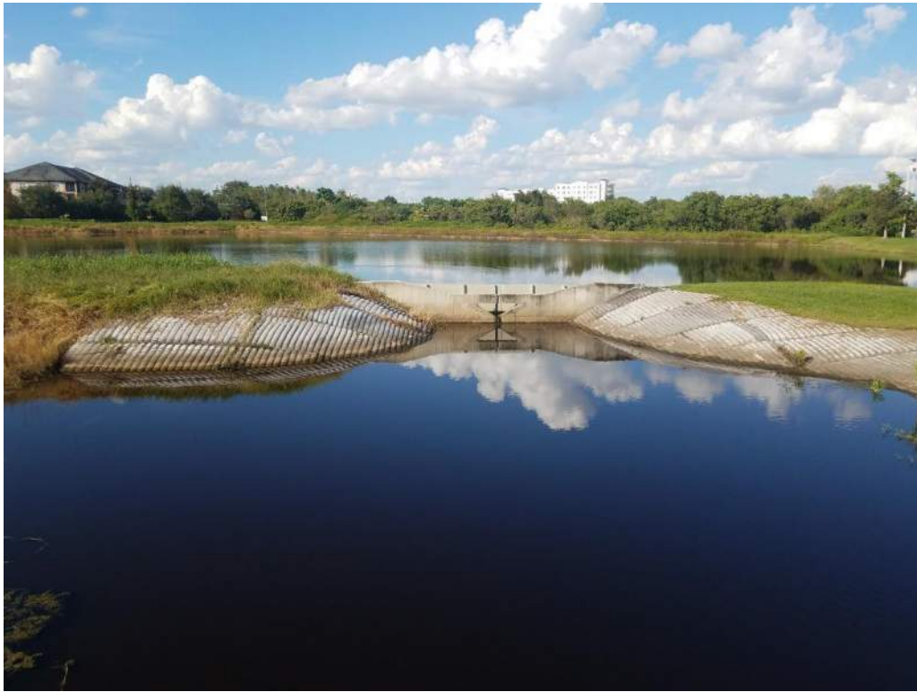
Weir connecting Partin Promenade stormwater pond to Fennel Slough canal. Facing north from Pedestrian Bridge.
