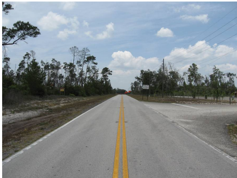
Photo 5.2. Looking east at Old Melbourne Highway (8OS2564) which forms part of the southern boundary of the Conservation Area. Note modern ditches, elevated shoulders, and road bed. Also note modern pavement has replaced original red brick.
