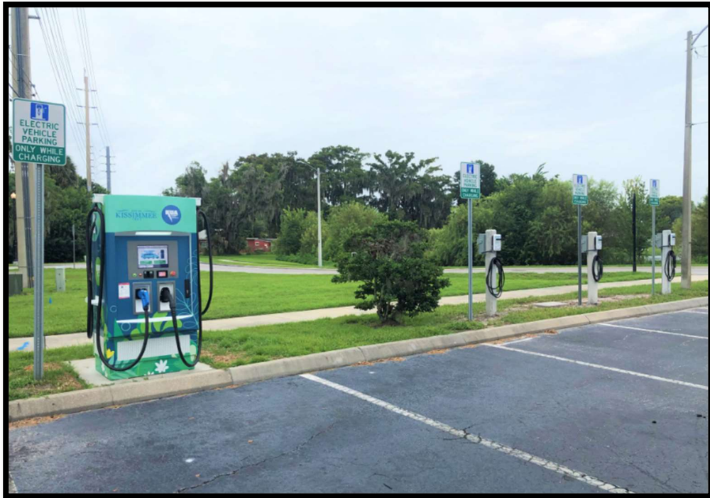
Figure 11: EV Charging Station Hub at Kissimmee Civic Center 13
